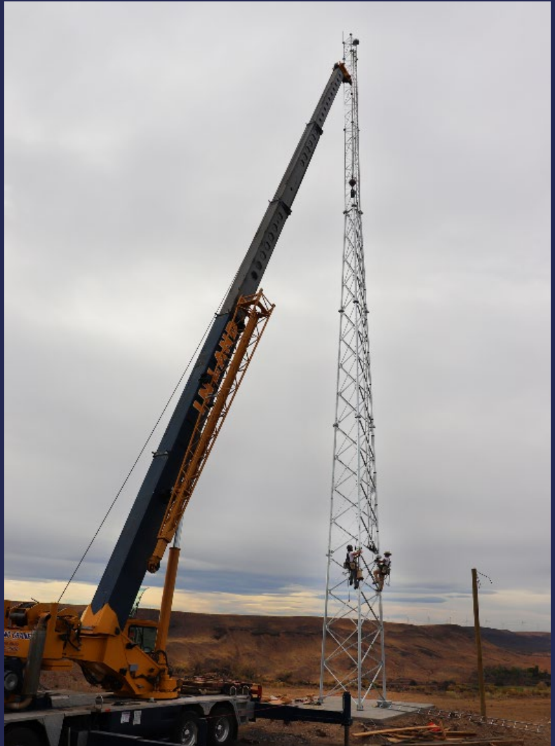
Photo Above: Construction of a Broadband tower in Bliss courtesy of White Cloud Communications.
